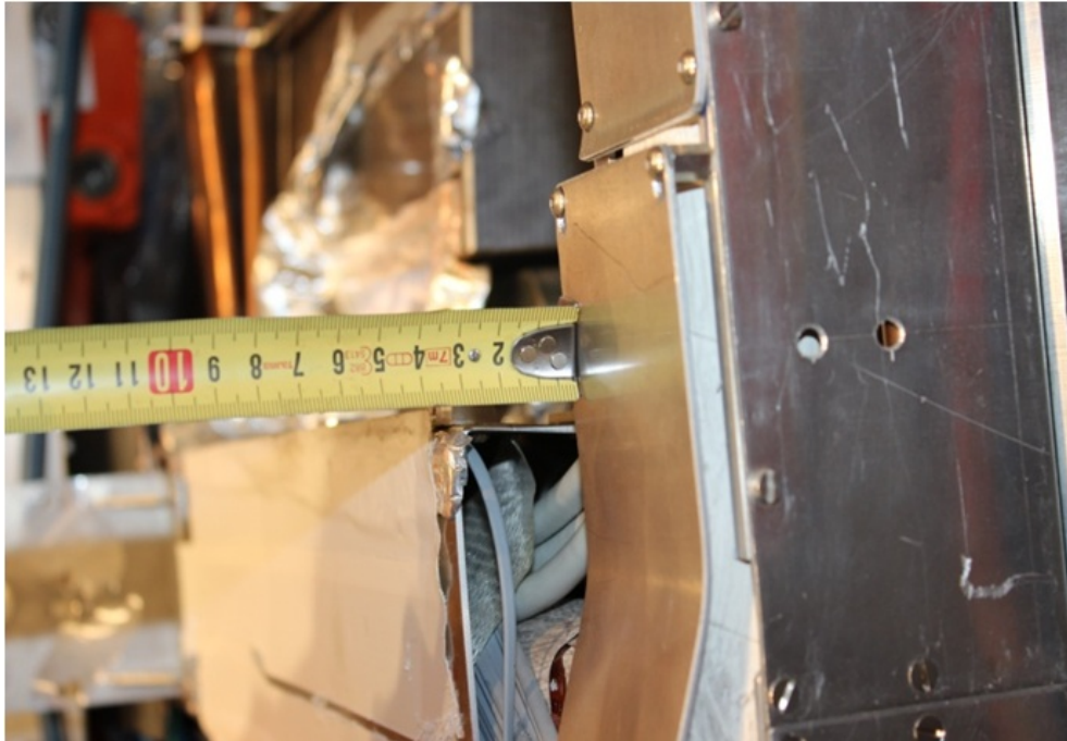
Figure 7.9: The maximum clearance available to place the cables from the CSC to the GE1/1 patch-panel.
