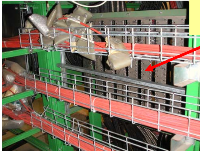
HV Patch Panel
