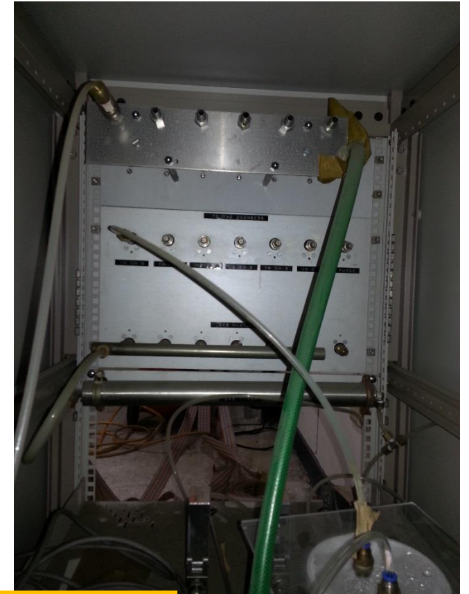
Rear View showing humidifier and mixing volume
