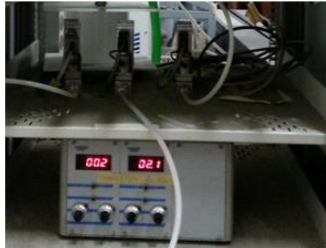
3x MFCs with plastic piping
