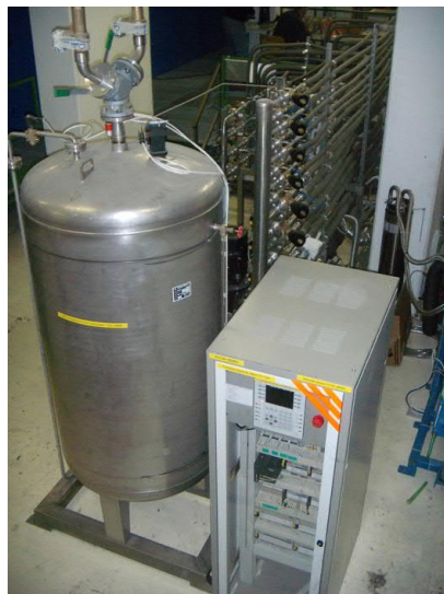
Figure 8.2. PLC/Electrical rack and tank.
