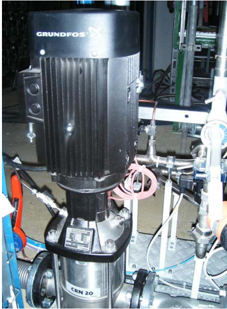
Fig. 6.2.1 – Pump and containment valve
