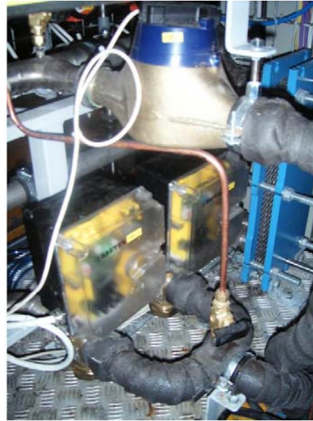
Fig. 6.2.2 –Heat Exchanger, regulation valve and flowmeter
