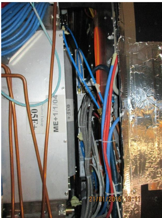
Moving up to last RE1/1/04 tight up against ME1/1/04. Signal cables are connected. No chamber "above"
