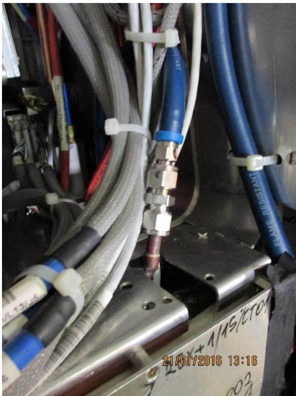
Close look at cooling unions
