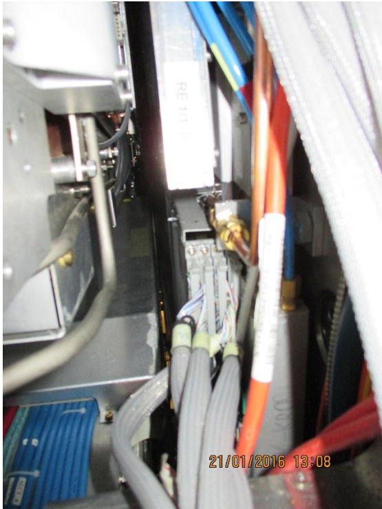
View of RE1/1/01 patch panel and RE1/1/02 chamber structure with copper cooling lines. In addition the Soft Blue gas lines are visible.
